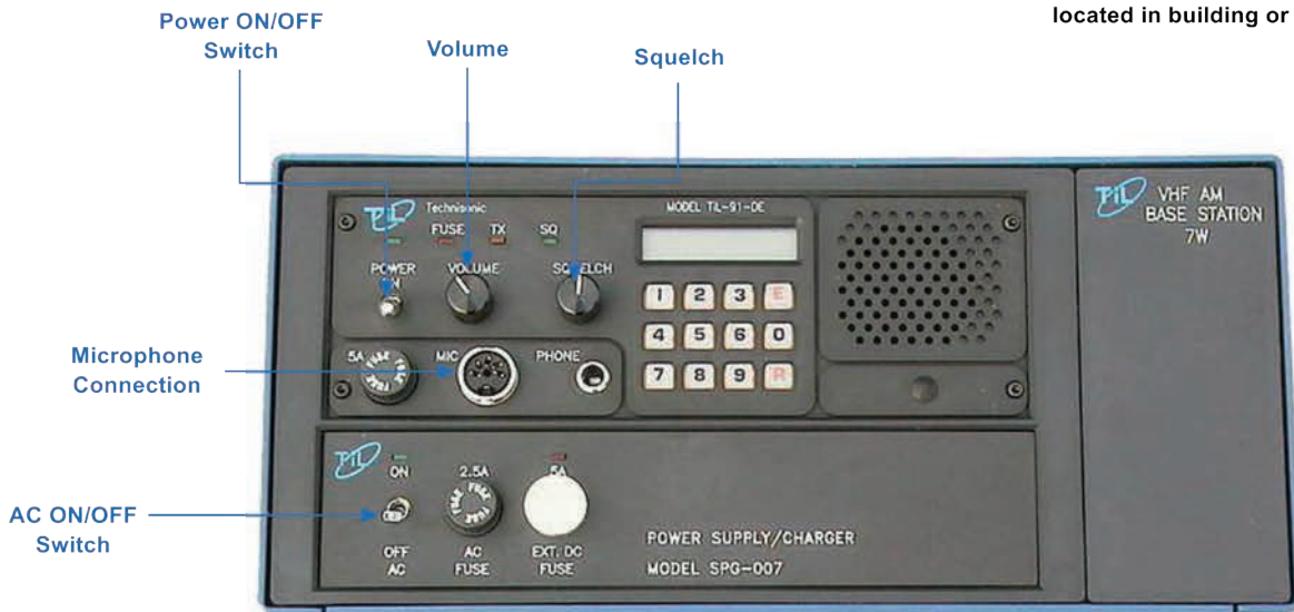
Figure 2: TBS-150 Base Station (Located in building or Tent)
